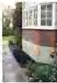
acceptable light well
